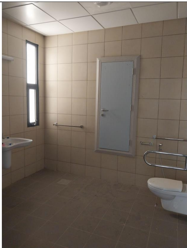
Accessible toilet (Jordan University of Science & Technology, Jordan)
