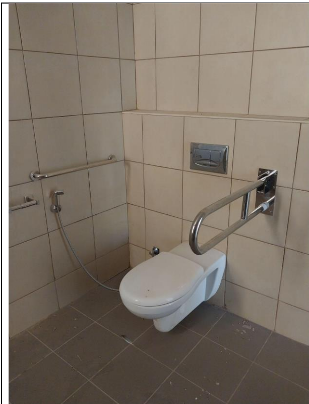
Accessible toilet (Jordan University of Science & Technology, Jordan)
