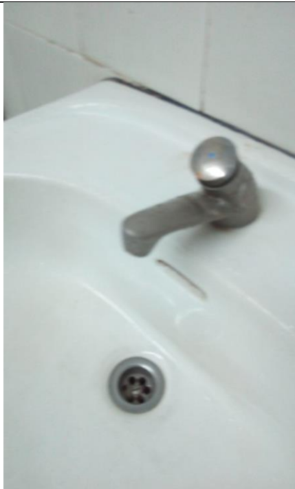
The system of self-locking washbasins is adopted and is calibrated to control the operating time and the amount of water flow (JUST, Jordan)
