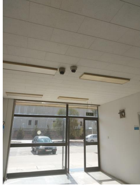
cctv system example
