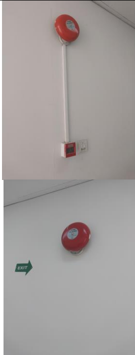
FireAlarm System and in BMS buildings it connected with the applications and monitoring
